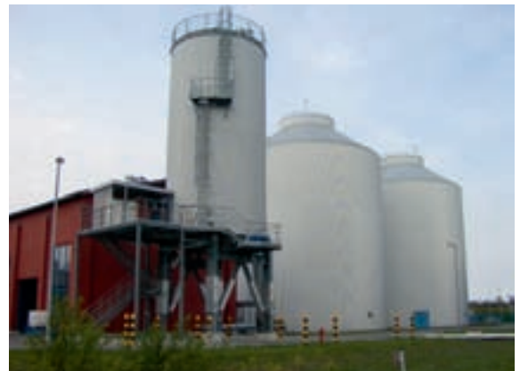
Sewage plant Wansdorf
