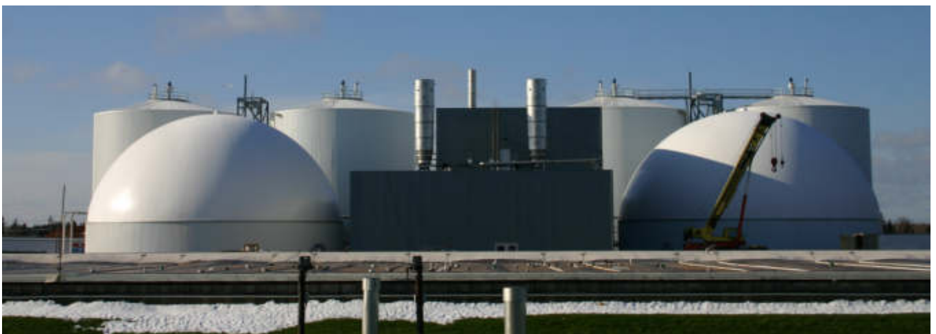
Biogasanlage in Kanada Biogas plant in Canada
