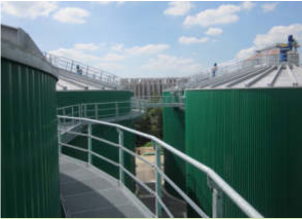
Biogasanlage Dorsten 8 Fermenter mit jeweils 3.200m 3 Biogas plant in Dorsten 8 fermenters, each with a capacity of 3,200 m 3 .
