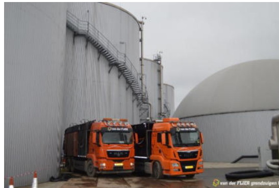
Abtransport Sand/Schlamm mittels Saugwagen / disposal of sand and mud by suction truck
