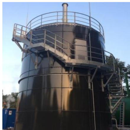
Trittau treatment plant Low pressure gas depot 30 mbar Volume: 250 m 3
