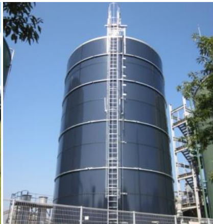
Nantan treatment plant (Japan) Unpressurised gas depot Volume: 500 m 3
