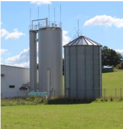
Vestenbergsgreuth treatment plant Unpressurised gas depot Volume: 200 m 3
