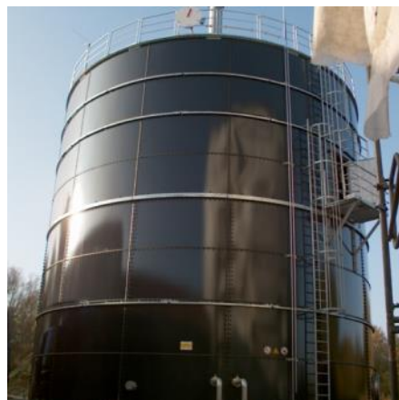
Rietberg treatment plant Low pressure gas depot 50 mbar Volume: 1,000 m 3
