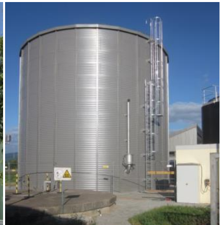
Edenkoben biogas plant Unpressurised gas depot Volume: 1,200 m 3
