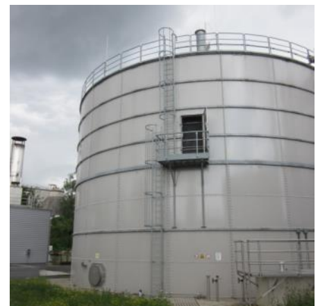
Wiesbaden-Biebrich treatment plant Low pressure gas depot 45 mbar Volume: 2,500 m 3
