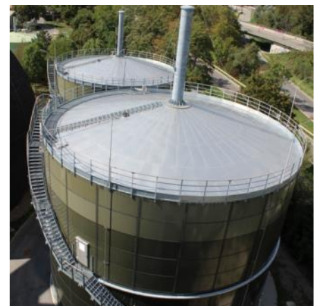
Mainz central treatment plant Low pressure gas depot 55 mbar Volume: 2,500 m 3 and 3,700 m 3
