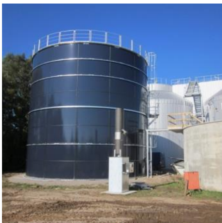
Nordhorn treatment plant Low pressure gas depot 50 mbar Volume: 1,000 m 3
